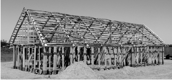
Figure 2a. House 2 under construction on the historical site. The characteristic wall construction can easily be identified.
