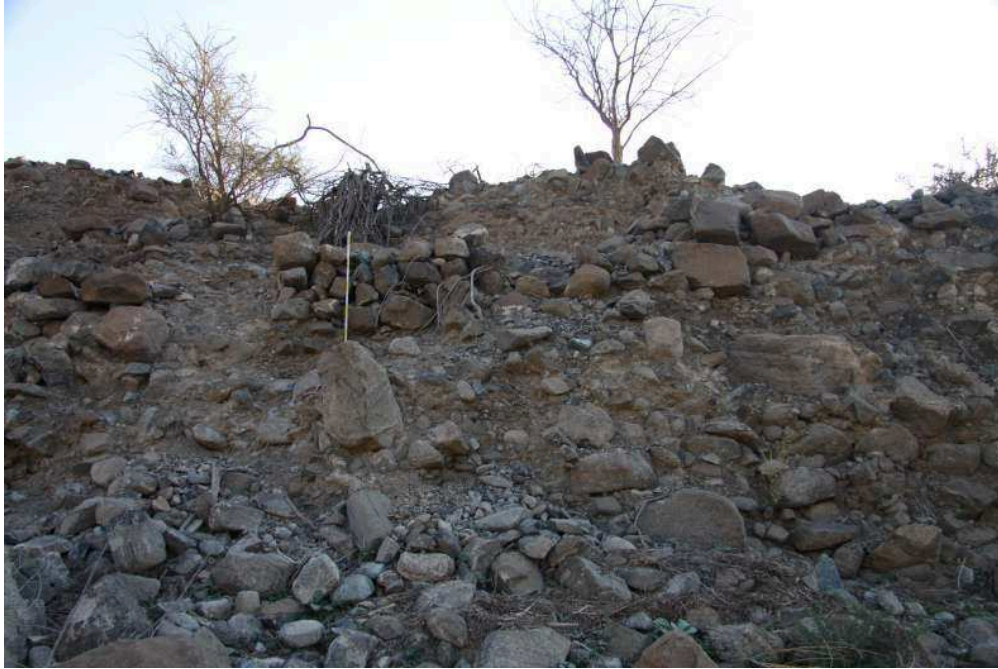
Figure 5.69: Side wall of the upper ramp before reconstruction (situated at arrow B in Fig. 4.68).
