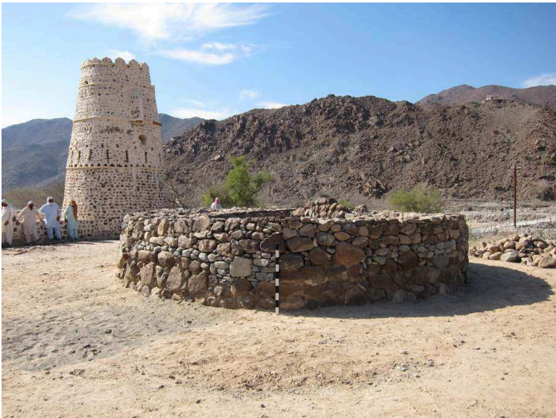
Figure 5.63: The UaN tower after partial reconstruction in 2011. The grey wadi pebbles separate the original wall from the reconstructed part above. Reconstruction appeared necessary in order to protect the preserved basic structure of the Bronze Age building.
