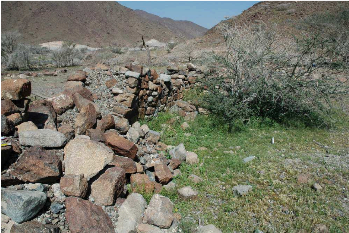
Figure 11.31: Feature 8 – tilted part of the wall.
