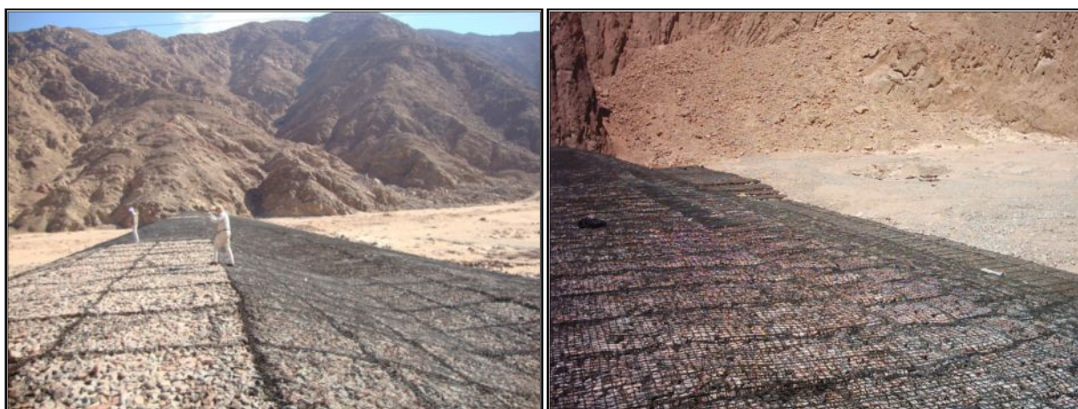
Figure 151: Protective Dam 1 at W. El Ghaieb Figure 152: Protective Dam 2 at W. El Ghaieb
