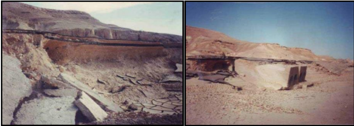
Figure 3: Some of Destructive Effects of Runoff on Infrastructure in W. Dahab
