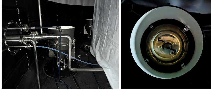
(a) Bottom veto PMT of OSIRIS in front of the connection flange of the LHS to the steel tank. Eight such PMTs are installed in the outer volume around the PMT frame. Picture taken in August 2023 by T.Sterr.
