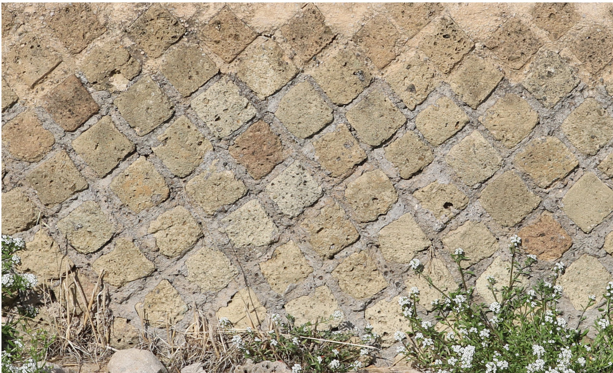
Fig. 7. Opus reticulatum facing from the so-called Villa of Tiberius at Sperlonga in Latium (second half of the 1st cent. BC) (photo by D. Maschek).
